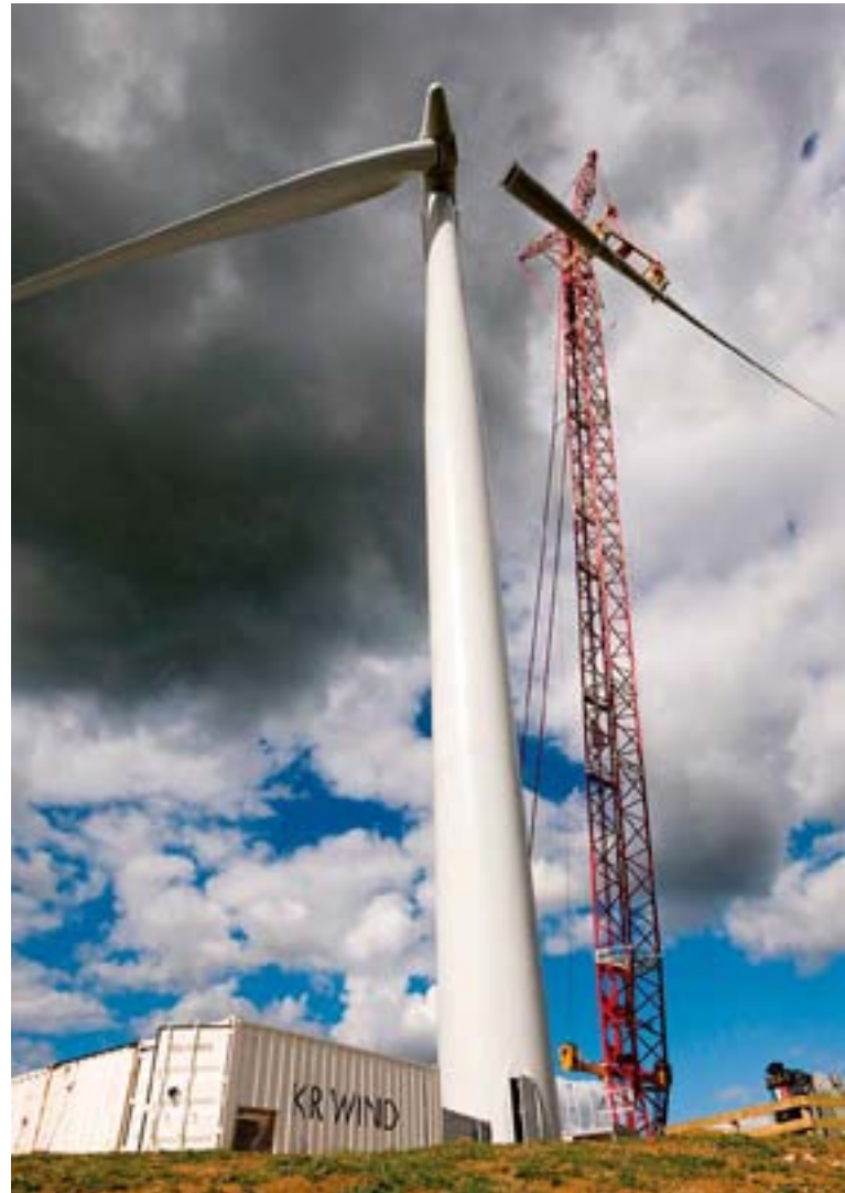
Te Uku wind farm, Waikato © Meridian Energy
